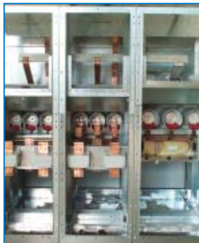
Excellent cabling and service access.
