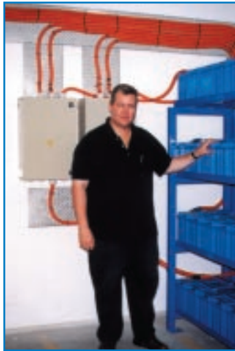
Battery backup at United Energy.
