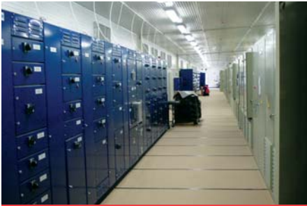
Prominent Hill Switchroom
