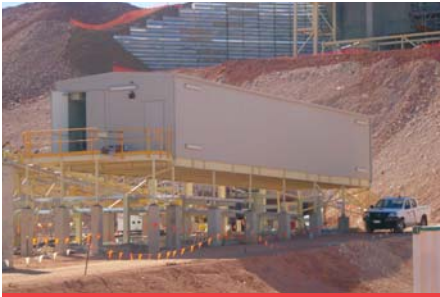
Switchroom at Prominent Hill site
