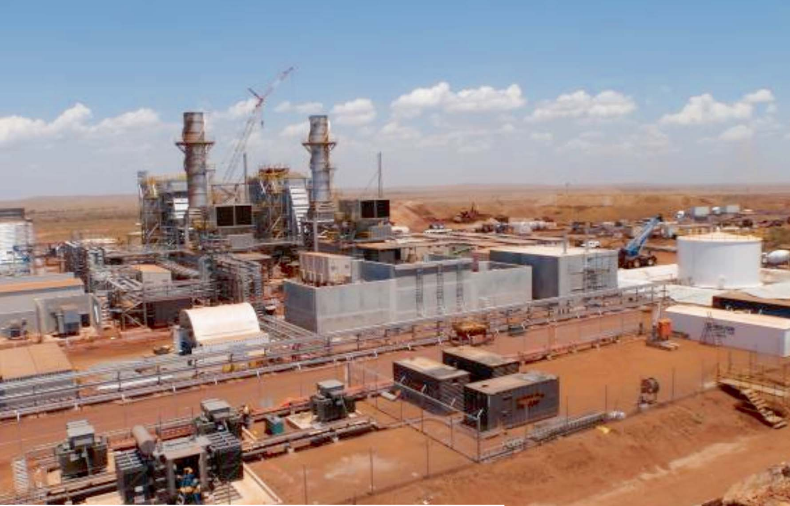
450MW combined cycle power plant for the Sino Iron Project
