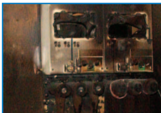
HV Protection no longer
