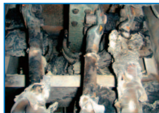
Typical arc damage
