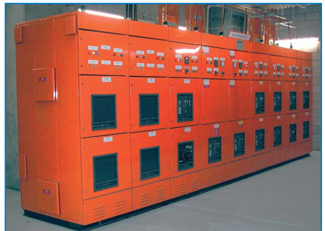
Very Dangerous If Not Serviced
