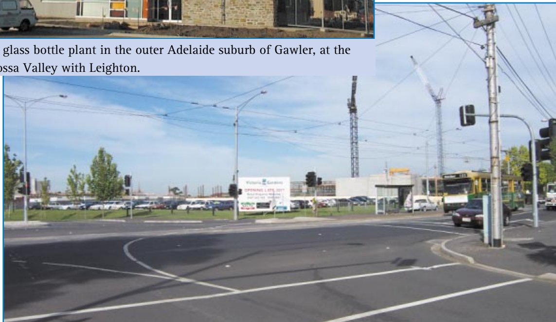
Victoria Gardens shopping and commercial precinct in the inner Melbourne suburb of Richmond. A major new project with Probuild.
