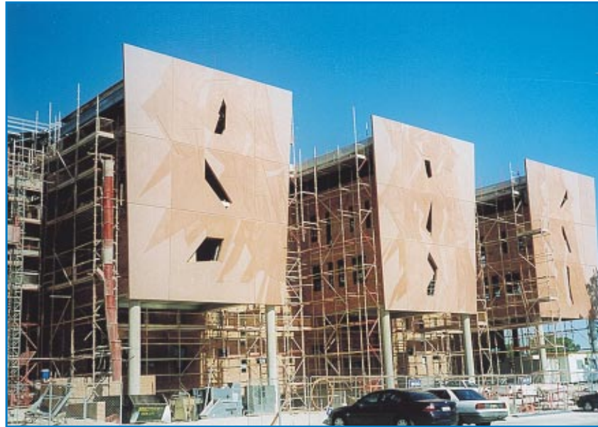
The Curtin University Business & Physiotherapy School in the Perth suburb of Bentley. A major new project with B.G.C. Constructions.
