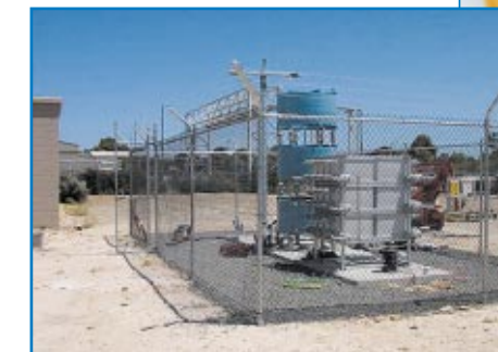
A 22kV Outdoor PFC unit
