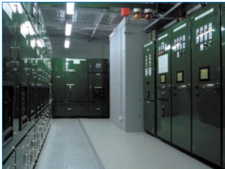
High density power distribution, a feature of our N Series switchboards
