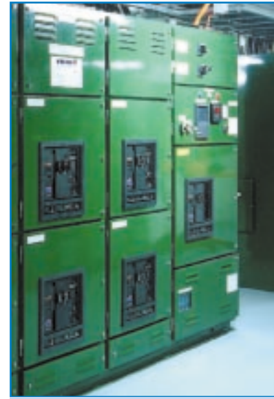
Main and standby supplies arranged
